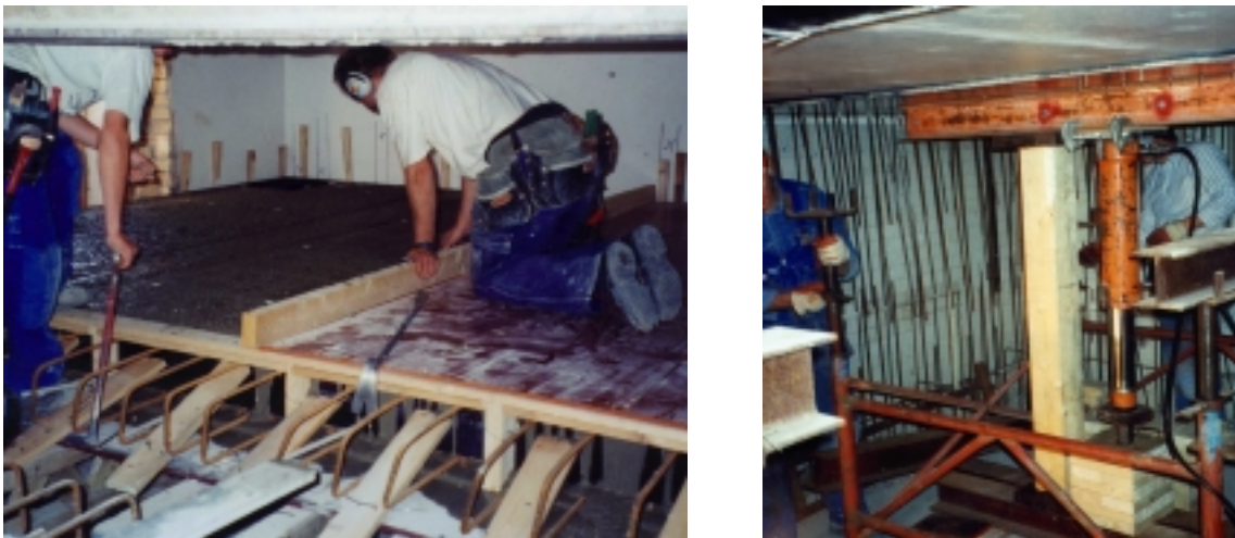
Figure 1.2 Casting and lifting of roof slab in civil defence shelter inside an existing building.
